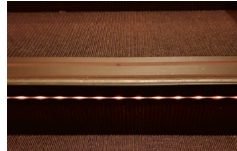
► Stair light mounted in stair nosing, shining down along the risers.
